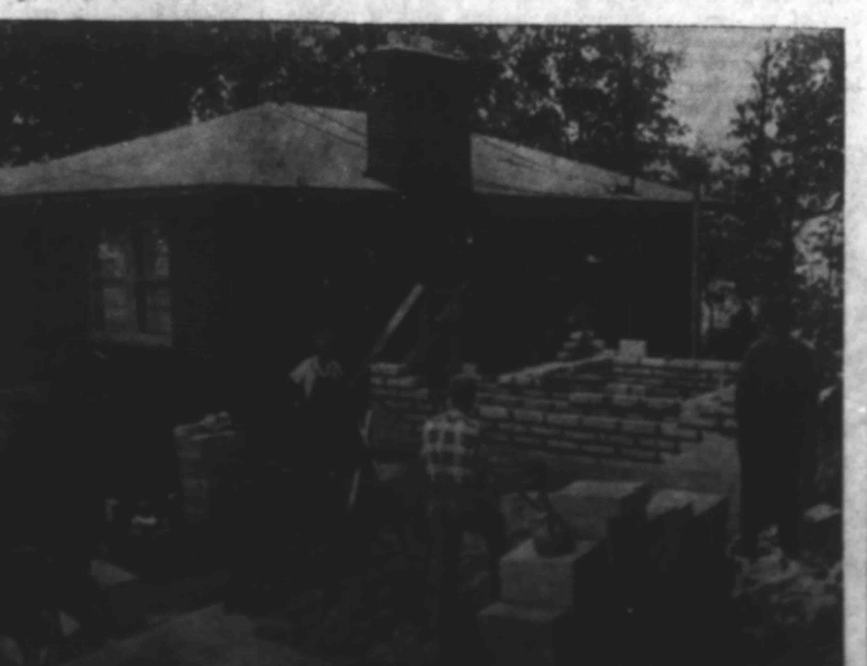
GUEST HOUSE—Frank Twyman, civil defense radiological officer for Tennessee, has perhaps the United States' only guest fallout shelter. Twyman, who has a family shelter in the basement of his home (background) in Nashville, is constructing a shelter for friends in his back yard. Twyman said his main reason for building the second shelter was to show people the proper way to build this type and show actual costs and specifications.
